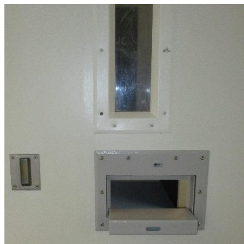
Image 23: Photo of a cuff trap and viewing window (external). As well as CCTV, these provide staff oversight while young people are in rooms
